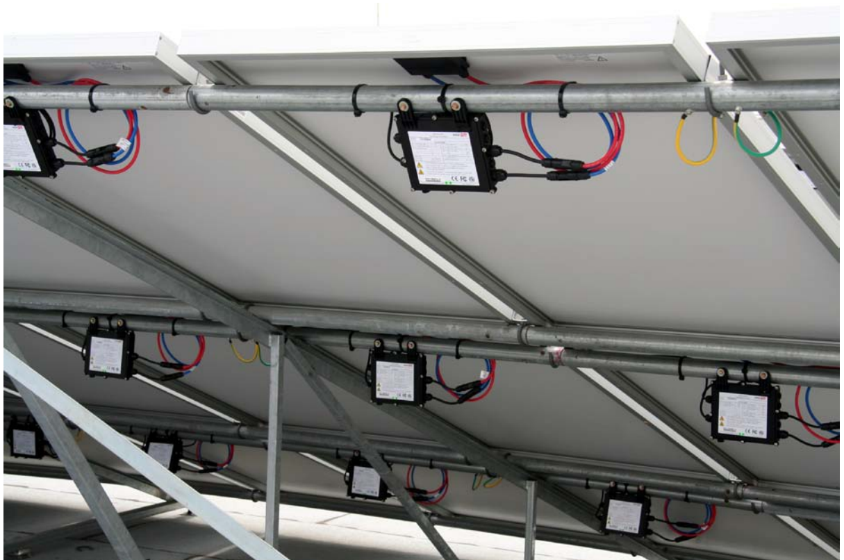
Figure 1: 100 kW Installation – Inverters (photos courtesy of SolarEdge)
