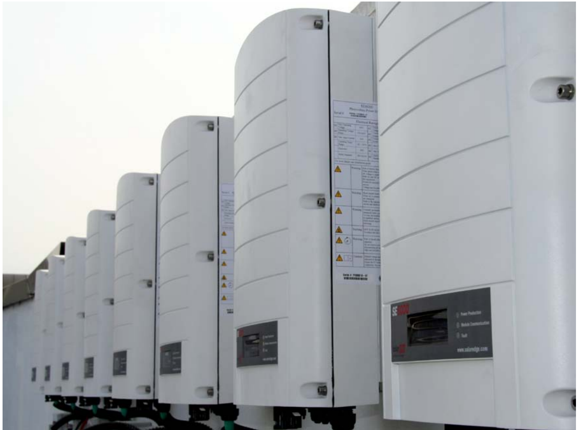
Figure 2: 100 kW SolarEdge Commercial Installation (photos courtesy of SolarEdge)
