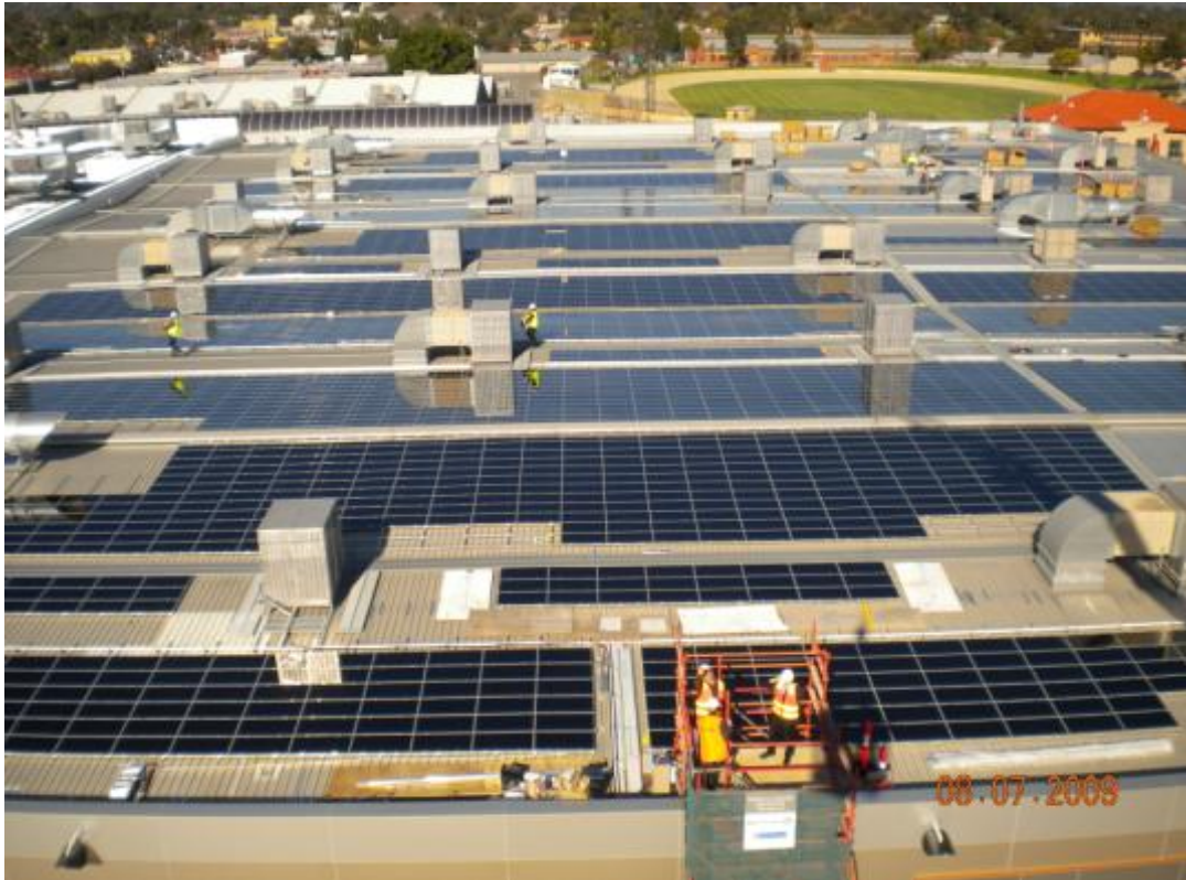
Figure 6: 1 MW PV array on Adelaide Showgrounds (Photo: Solarshop)
