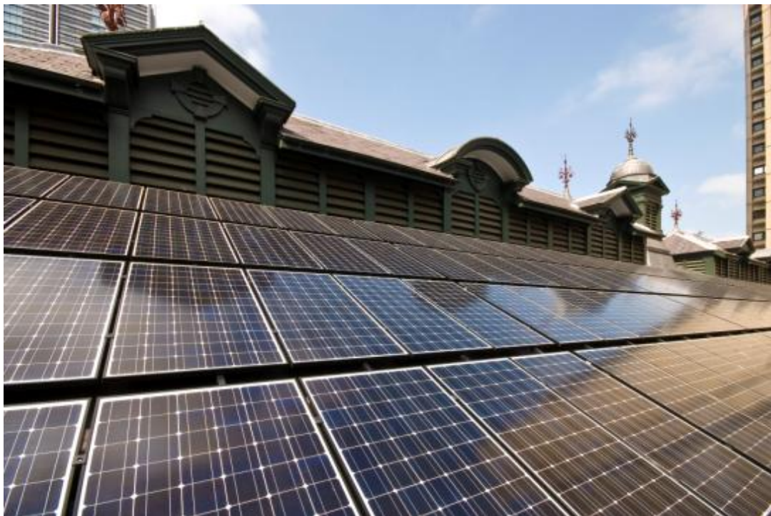
Figure 1: 48 kWp PV array on Sydney Town Hall (Photo: NSW Government Architect's Office)
