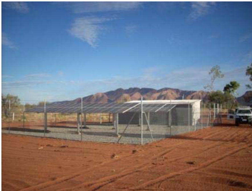
Figure 1: 48 V Bushlight system at New Bore, Northern Territory Photo: Bushlight
