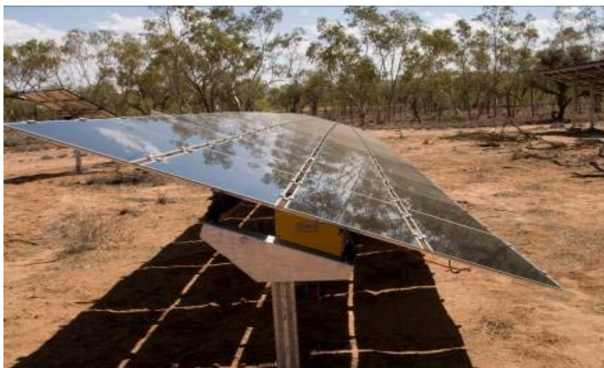
Figure 3: CdTe array at Desert Knowledge Australia Solar Centre. Photo: S. Troman.
