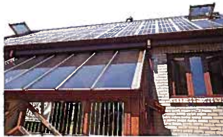
The UK's experimental programme will help to assess the impact of connecting numerous small embedded generators, like the one from Oxford UK shown here, to the mains grid.
