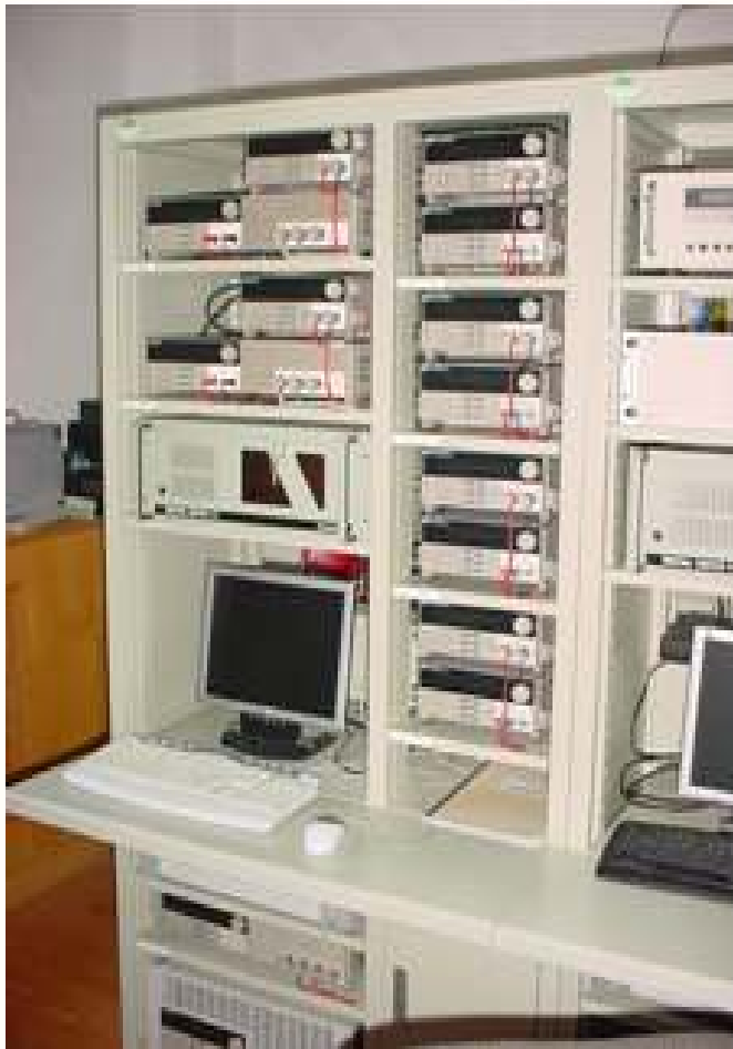
indoor test system
