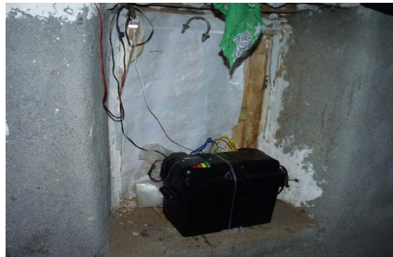
Figure 3: Poorly installed PV system
