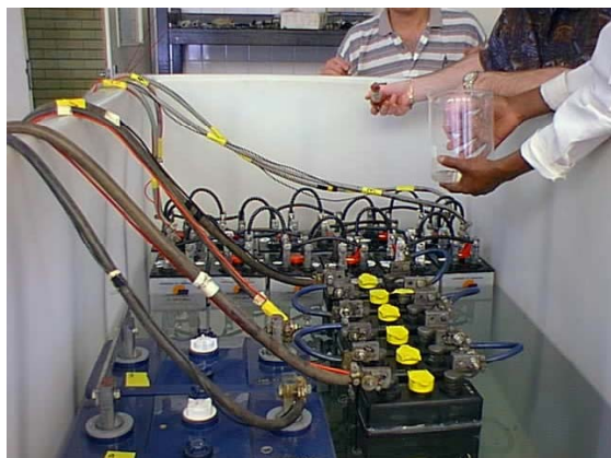
Figure 2: Acceptance testing of batteries in Southern Africa
