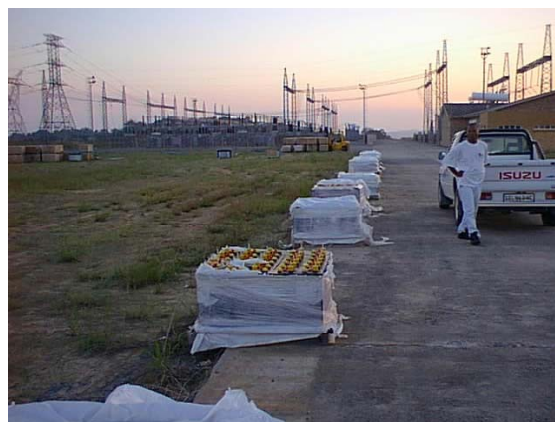
Figure 1: Incorrect storage of batteries
