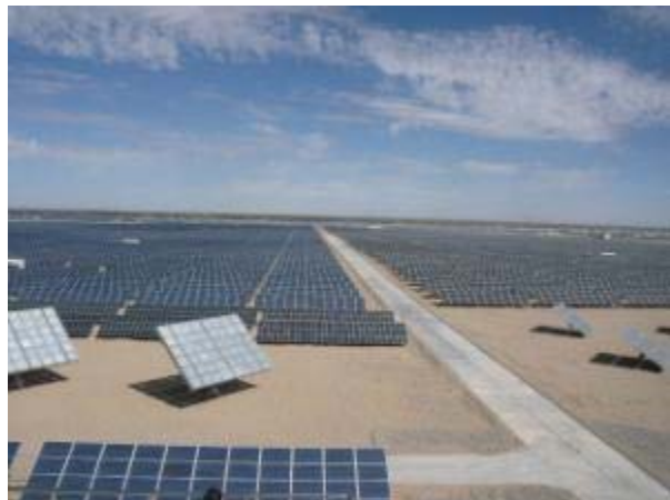
Yellow River hydroelectricity, PV power station : 300MW (planned to expanding to 500MW)
