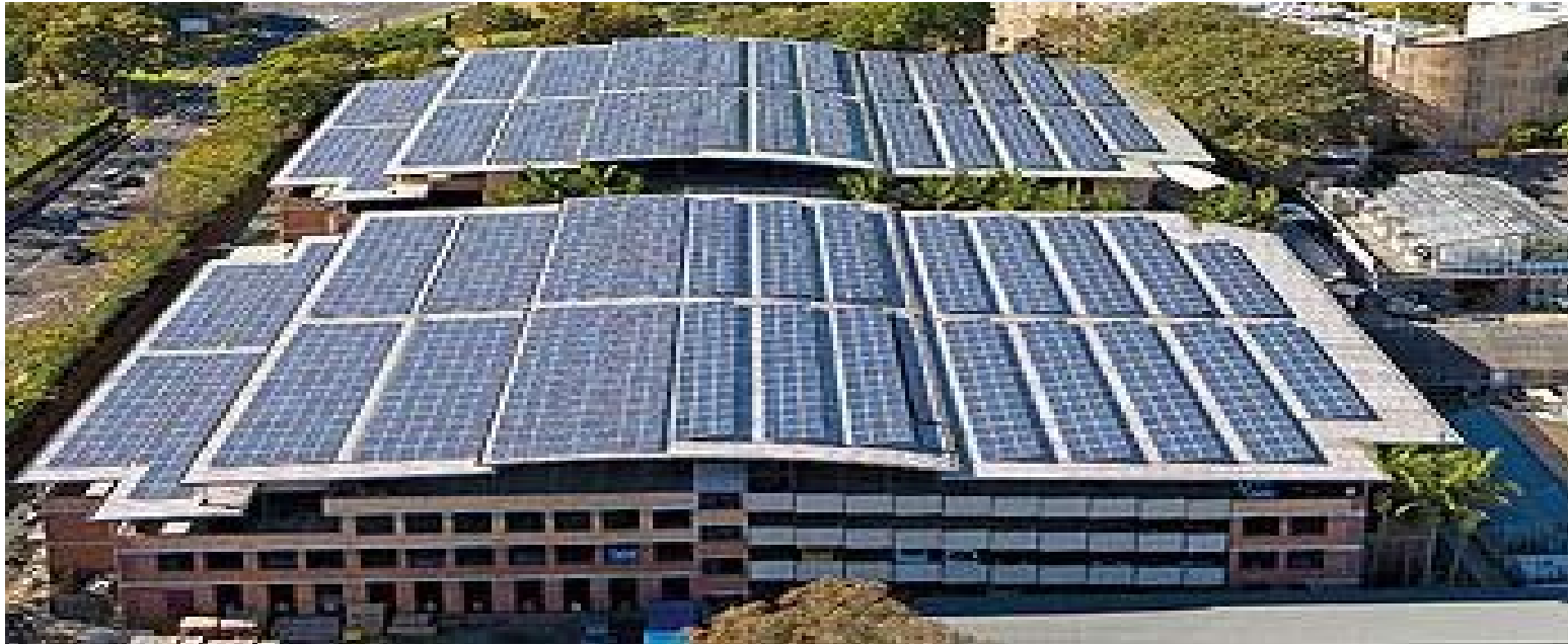
1.22 MWp PV system, University of Queensland
