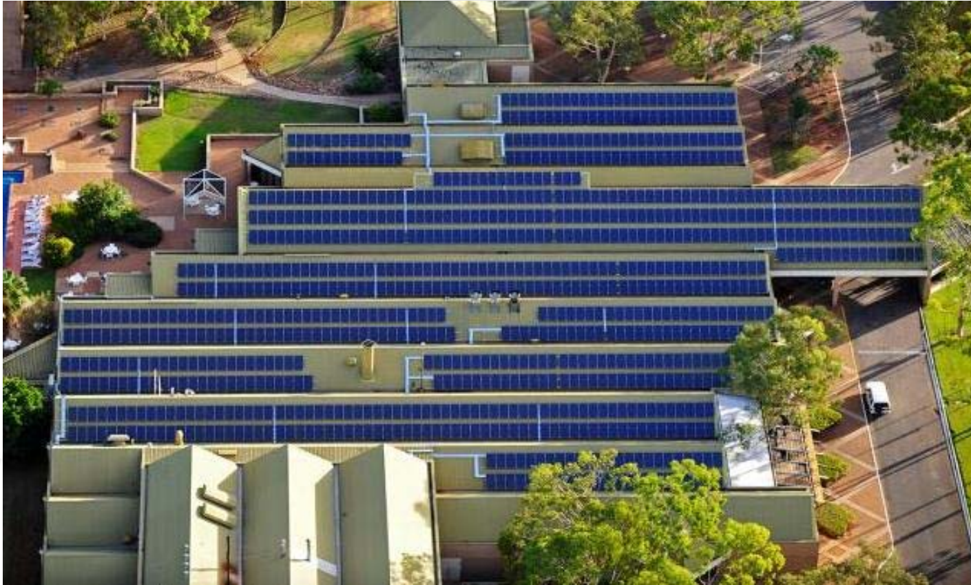
305 kWp PV system on Alice Springs Crown Casino Photo: SunPower Corporation
