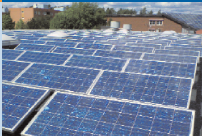
Fig. 2 - 64 kWp PV system on the roof of Andersberg Centrum and on the triangular roof of the nearby Andreas' Church in Gävle (photo Anders Holmsten, Gavlegårdarna).
