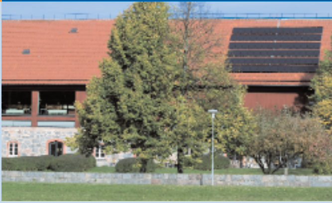
Fig. 3 - The system is the first in Sweden with CIGS modules from Solibro, a company that was founded as a spin-off from thin film research at Uppsala University. The system is installed at the Swedish University of Agricultural Sciences in Uppsala (photo Julio Gonzalez, SLU).
