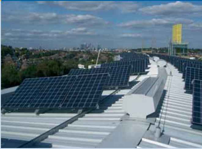
Fig. 2 – 13,7 kW PV array at Lewisham Hospital, London (photo Dulas).
