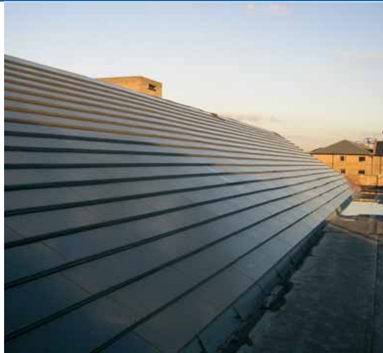
Fig. 1 - The 23 kW solar roof at the Print House in Dalston, East London is the largest PV roof tile installation in the UK (photo The Bootstrap Company).
