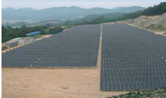
Fig. 4 - The 2,2 MW PV power plant installed at Munkyeong, Kyungpook Province in 2007.
