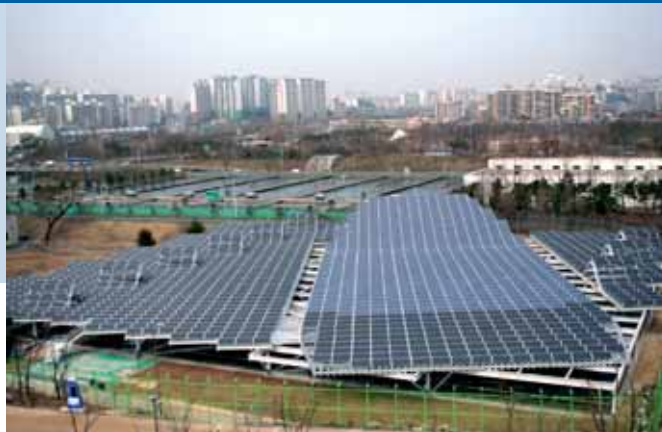
Fig. 3 - The 310kW PV power plant installed at water purification sites from Seoul Metropolis in 2007.
