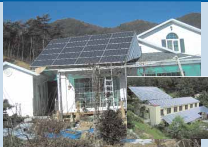
Fig. 2 - 3 ~ 5kW grid-connected PV systems on residential houses under the 100 000 roof-top program.
