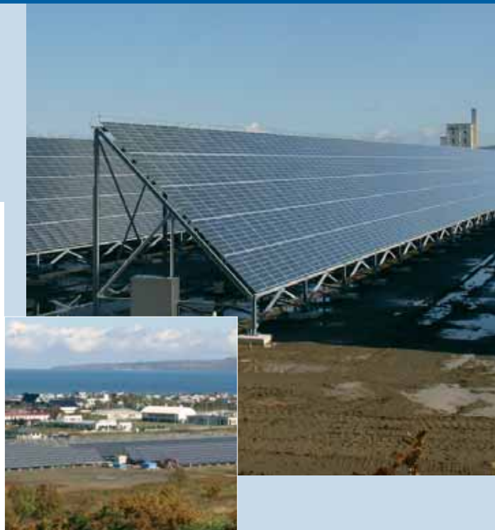
Fig. 3 - Wakkanai Photovoltaic Demonstration Facility (Under Constructed), 2 MW (end of FY2007), 5 MW (end of FY2010), Wakkanai-City, Hokkaido Prefecture (photo RTS Corporation).
