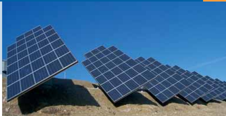
Fig. 2 – Italian Feed-in Programme: 50 kW PV plant in Brentonico, Trento (photo GSE).
