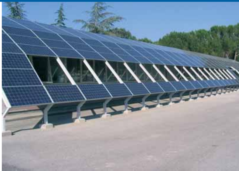
Fig. 1 – Italian Feed-in Programme: 40 kW PV plant in Narni, Terni (photo GSE).
