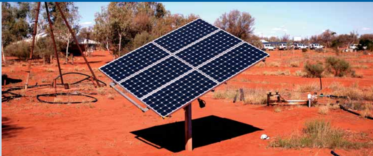
Fig. 1 – PV Water Pumping (photo S. Troman).
