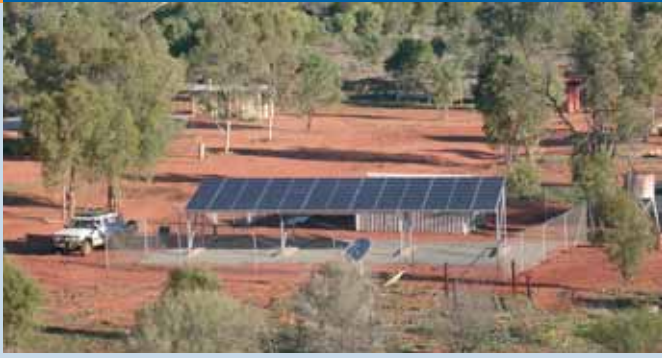
Fig. 3 - Bushlight community RE System installed at Wanmarra outstation in Central Australia.
